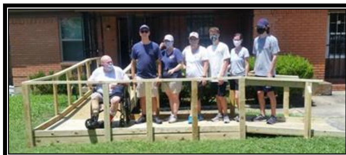
This 29-foot ramp was built on July 11 with two team leaders and 10 YMSL (North Dallas Chapter) volunteers, who provided 35 hours of labor.
